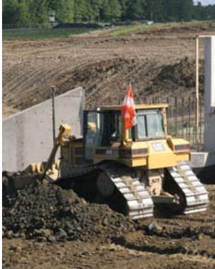
GPS-controlled dozers at the airport site proved so efficient that UCC had a machine restoring just 100 feet behind the machine making the lead cut.
